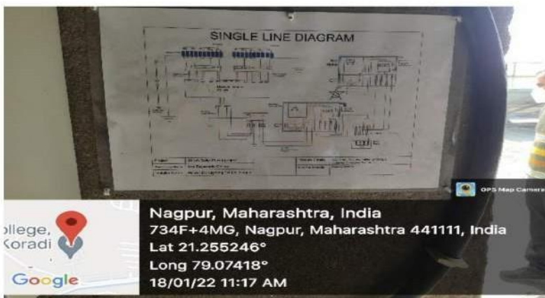
Junction Box and Net Meter
