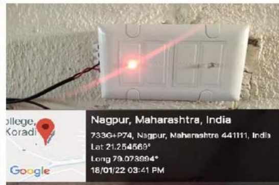
Sensor based lighting installed in college
